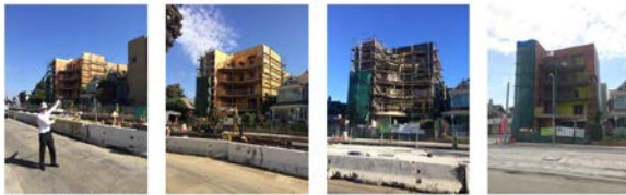
The Kaufmann Apartments at Step Up on Colorado - from start to finish!
